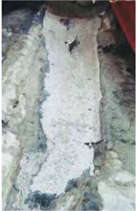
Fig. 14. Concave depression partially covered with plaster.
